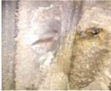
Figure 15: WW Hydrogen damage
