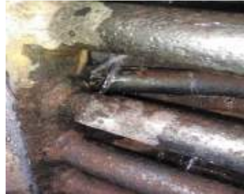
Figure 4 (a) SH Stub joint crack
