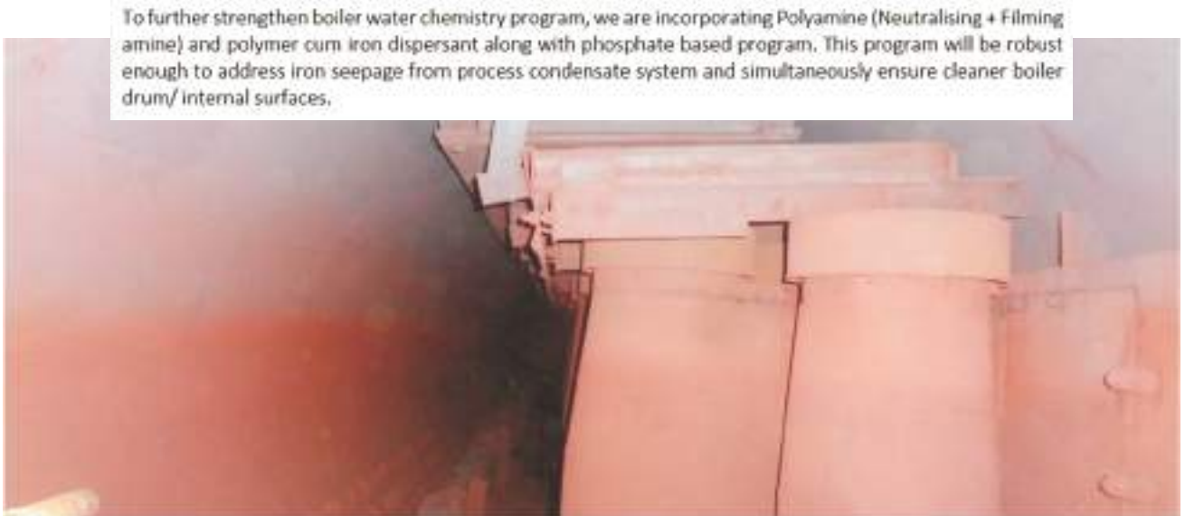
Photo 20: The above is a photo of steam drum in a paper mill with several boilers. The drum inspection revealed high level of iron dust. To facilitate online removal of iron deposit, polymer-based iron dispersant was introduced. Further filming amine chemical was added to protect the condensate touched surface to prevent online corrosion.
