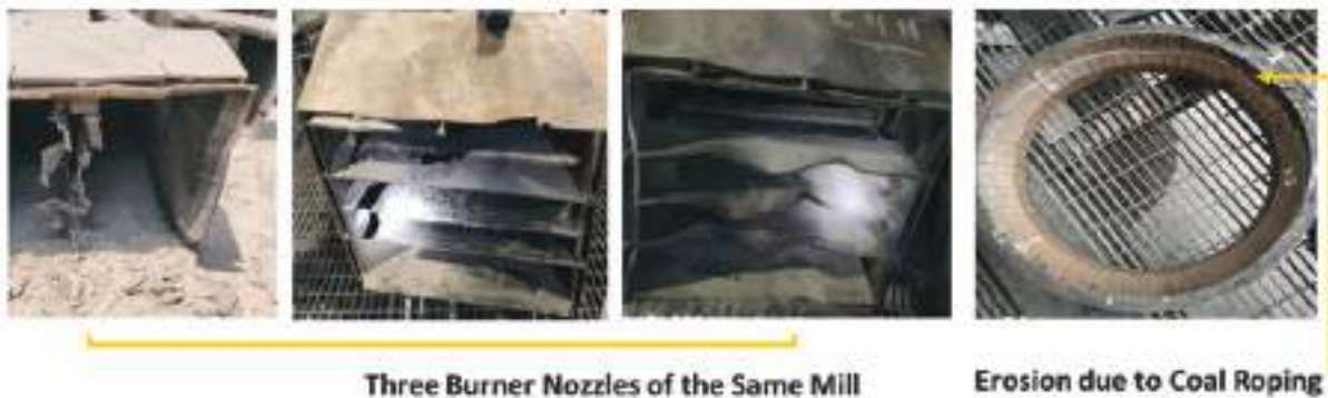
Figure 23: Improper air/fuel distribution across coal pipes
