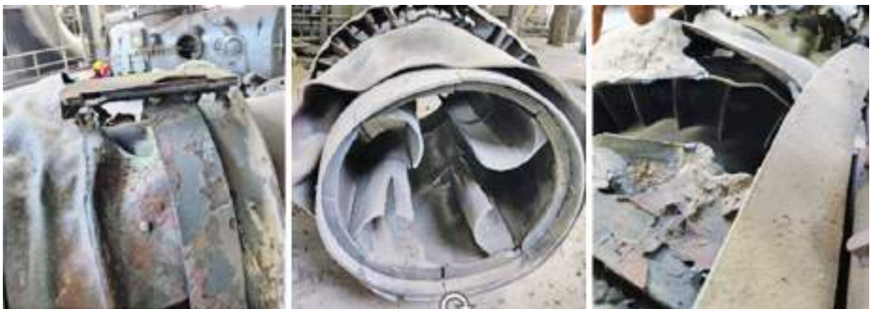
Figure 21: Damaged burners due to improper fuel/air distribution leading to non-optimal combustion
