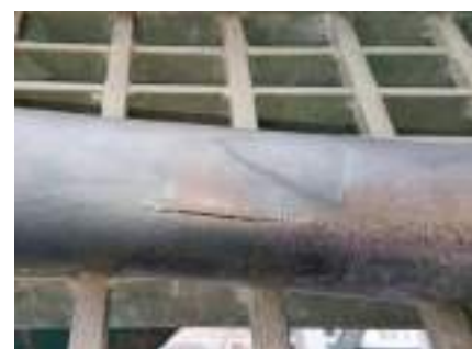
Figure 8: SH tube longitudinal crack
