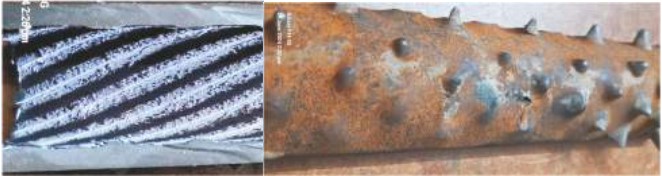
Photo 18 & 19: Two AFBC boilers with common TG underwent under deposit corrosion after the condenser tube leak incident. The boilers were run for more than a week after the condenser tube leak incident. Rifle bore tubes are sensitive to under deposit corrosion. The boiler had to be chemically cleaned.
