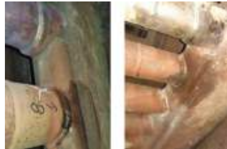
Figure 12: Attachment Weld failure
